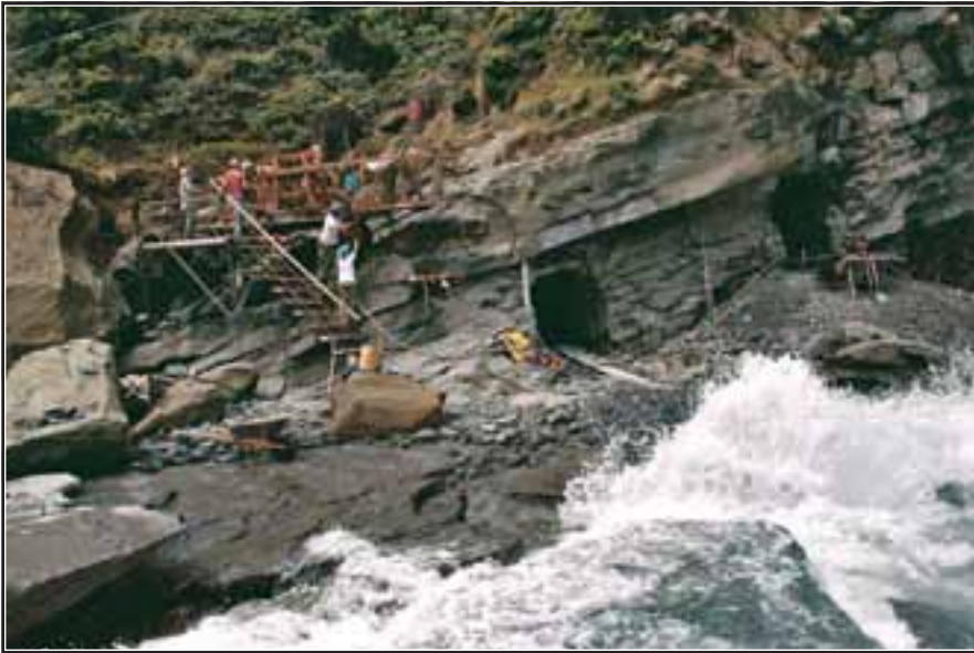
Positioned several metres west of the Slippery Rock tunnels and seemingly clinging to the rock face, a spidery-legged scaffold platform (above) built by volunteer Graeme O'Brien in 1989 proved to be strong enough to withstand the roughest seas. Accessed by a set of stairs, this structure was invaluable for storing equipment safely above the pounding waves of the Southern Ocean.
