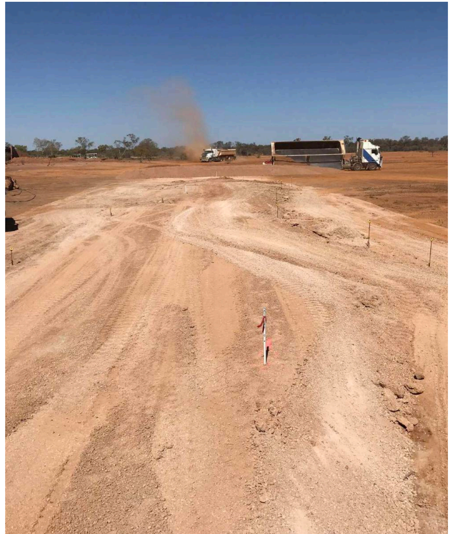
Building a pad out of compacted wet mudstone for the trackway at the Museum's Dinosaur Canyon. The yellow-topped pegs show the gravel height needed in order to replicate the base shape of the trackway in its original location.
